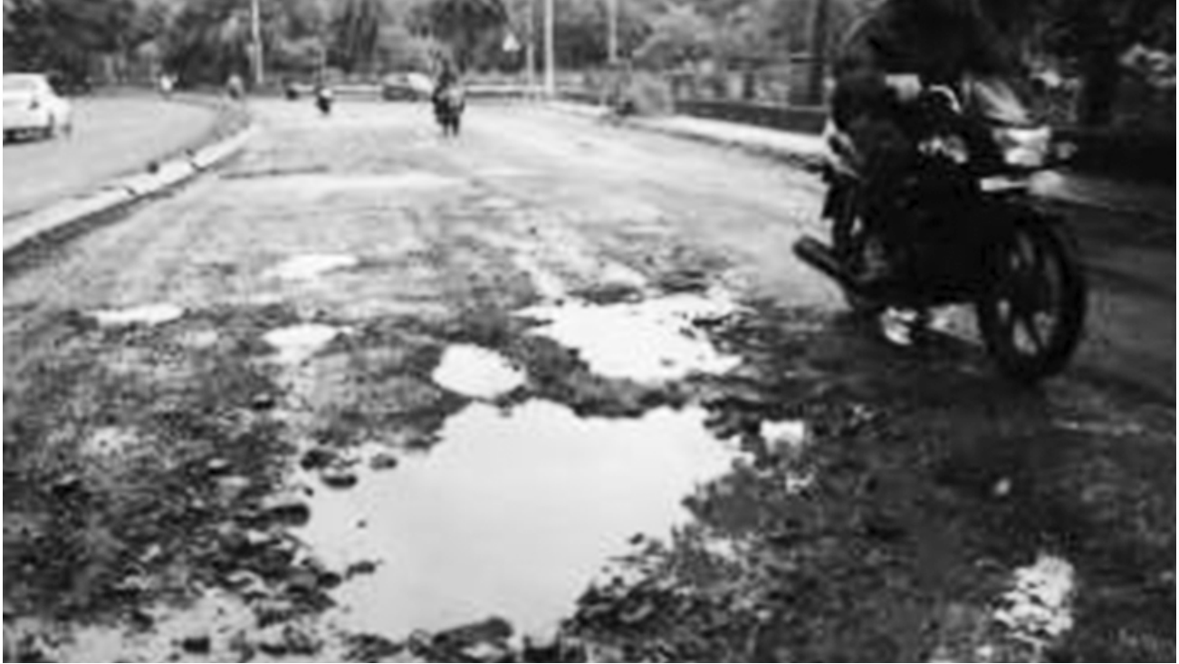
Fig. 1: Pothole on the Road Surface of Bengaluru (3)
